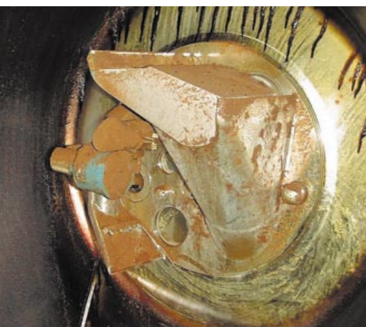
◀ Fig. 1 Process area of the centrifuge before CIP cleaning
